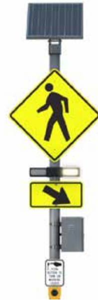
Rapid flashing beacon. Source TAPCO
